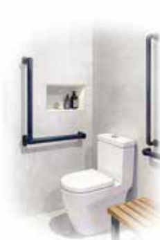
Grab Bars in Washrooms and Common Areas
